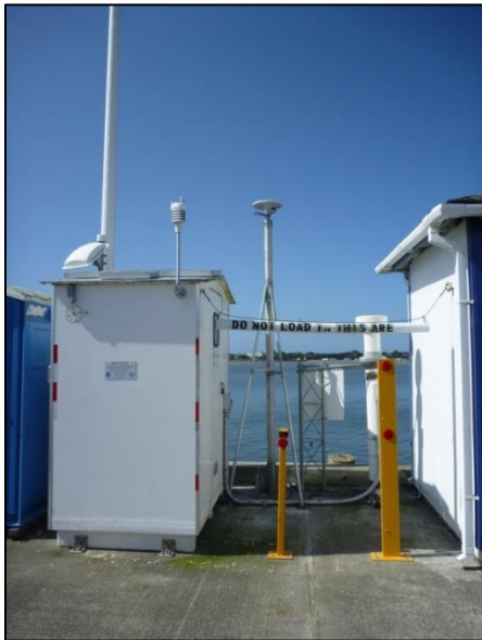
Co-located tide gauge and CORS GPS at Crescent City, CA
